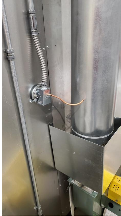
Exhaust Fan Air-Flow Tube Location
